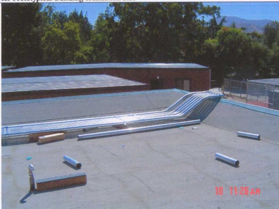
Rooftop installation of secondary electrical distribution
