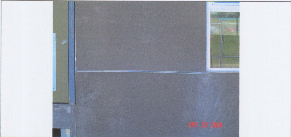
Low quality of plaster and joints application at prototypical classrooms. These are being corrected.
